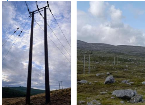
Photographs of typical wood poles in the landscape (Belltown Power, June 2026. NB: Belltown Power do not know how Scottish Power will choose to connect.)
